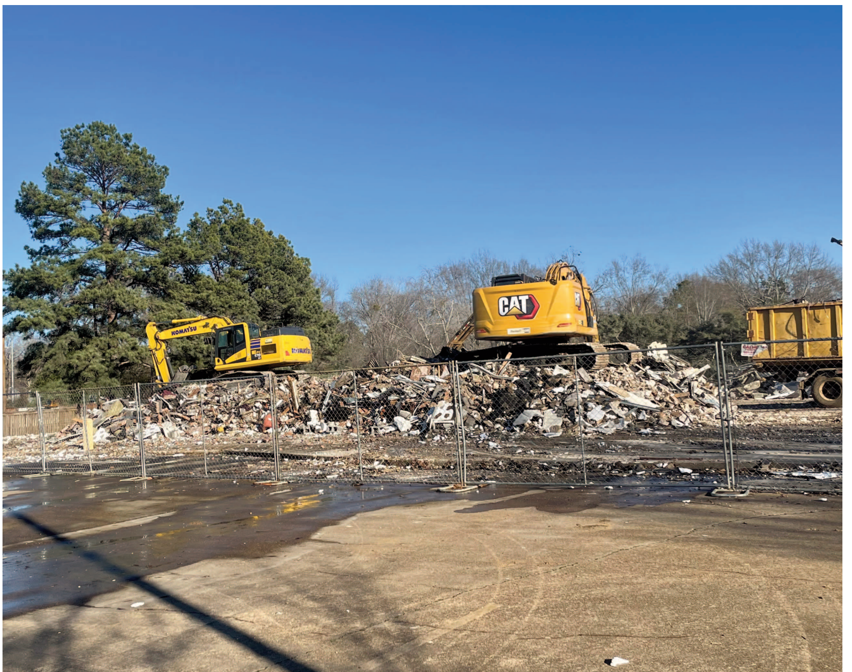
Crews tear down the former Ridgeland City Hall building located on U.S. Highway 51 weeks after a contractor accidentally tore down a section.
